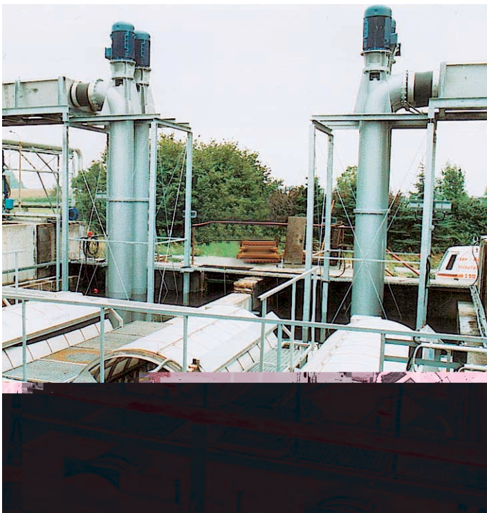
Pumps in a water recycling plant.
