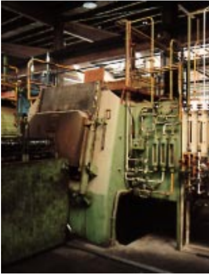
This gas heated Ipsen TQ-11 is equipped with 14 APM tubes, 83 mm outer dia and 1640 mm long. The tubes have been in continuous operation since December 1994 and none of them is exchanged.
