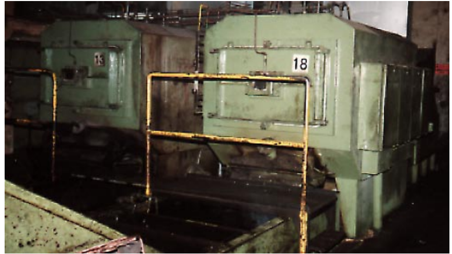
Two continuous hardening furnaces at 850°C with 6 Tubothal at 6.3 kW in the first zone and 6 at 4.2 kW. APM tubes 87 mm dia.
