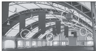
Air being moved in a circular pattern to heat an event tent.
