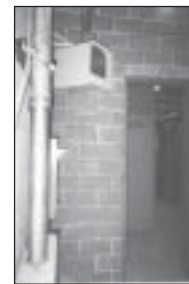
Freeze/Moisture Protection in a Generator Vault
