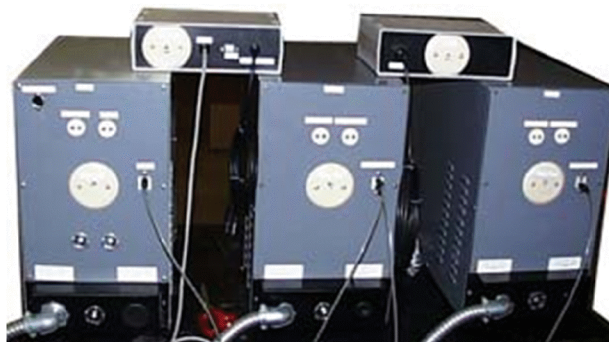
HIPAN-2010 control panel back. Typically customized.
