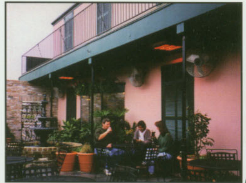
Infrared heating for outdoor restaurant seating comfort.
