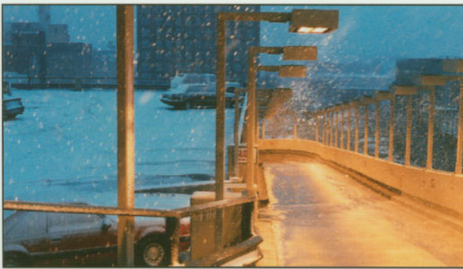
Infrared snow & ice control for parking garage ramps.
