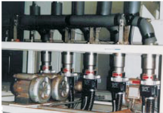
Five Heaters 5000 used to heat a tubular channel. Coated stranded steel wires are melted together as they are fed through the heated tubing.
